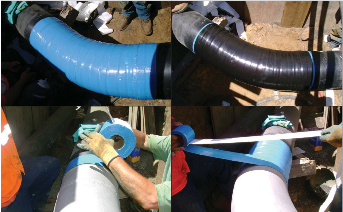
The above images show the proper installation of a field-applied pipe wrap and tape. Farwest Corrosion Control Coatings conducted the pipe repair during a relocation project in California in summer 2011.
